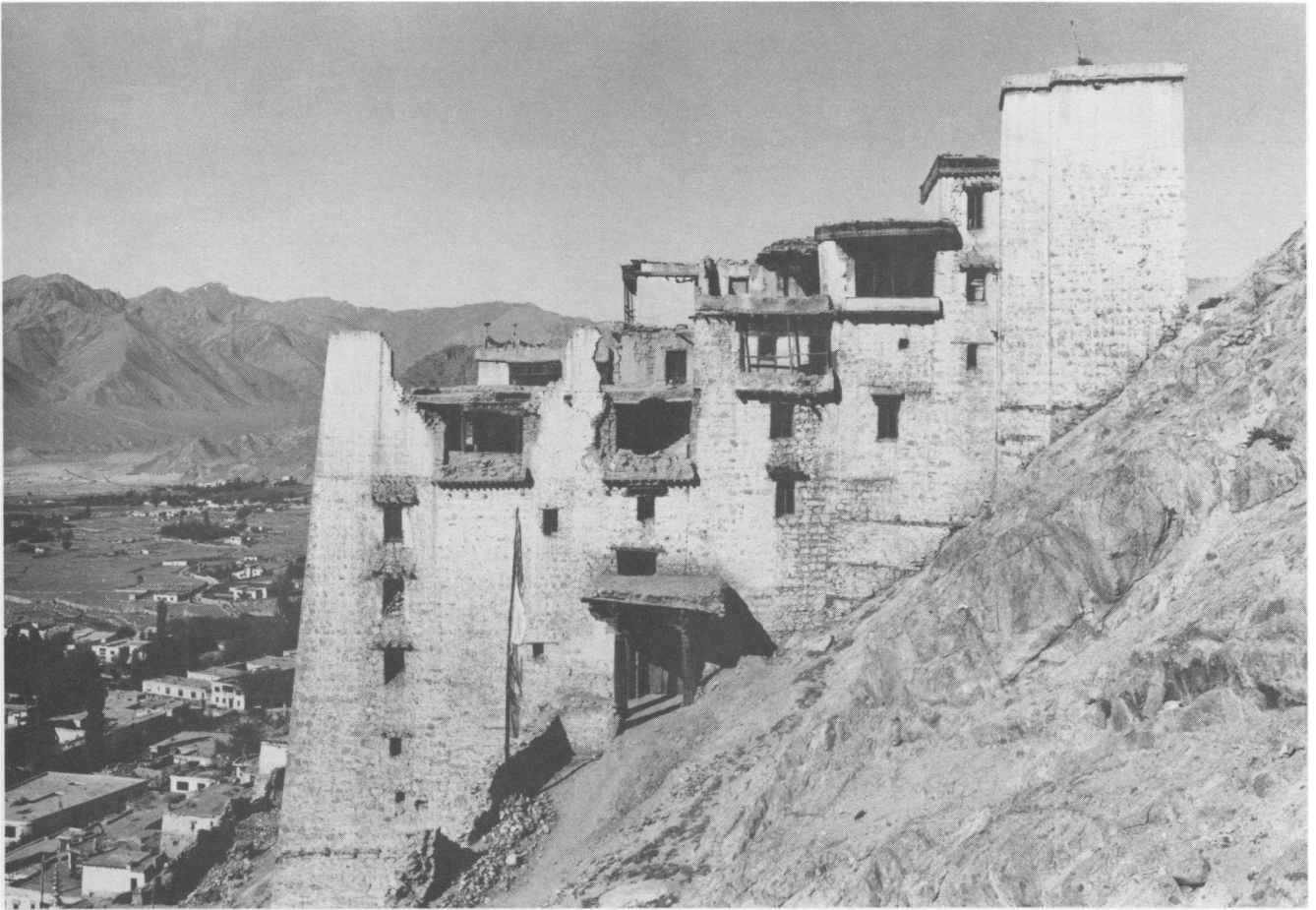
FIGURE 8. The east facade showing the main entrance porch. Note the present condition of collapse compared to Figure 3, the photo taken in 1930; most of the collapsed sections are in sun-baked bricks.
